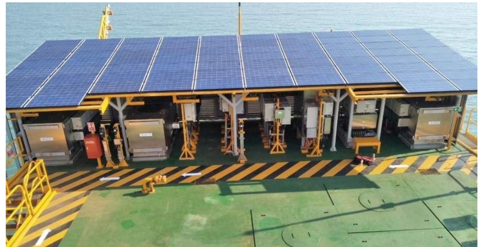
EPC contractor for 25kw Solar System (offshore platform)
